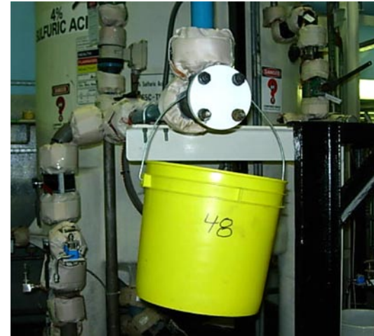
Figure 3-1. Blind flange with catch bucket
